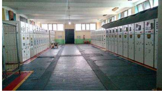
Gambar 1. Ruang Operational Kubikel Tegangan Menengah di Gardu Induk Titi Kuning.
